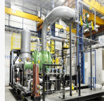
Process Gas System
